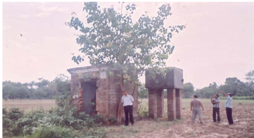
Damaged Pump house, Tube well not functioning but connected to Imamganj Branch Canal
